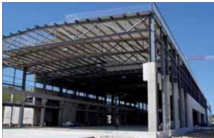
A purpose-built facility in Cadarache, France, will be used to wind some of ITER’s coils on site because they will be too large to be transported by road.
